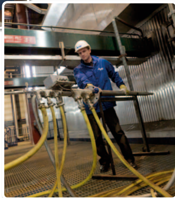
VTT has developed fouling monitoring services for multi-fuel boilers. By using VTT's methods, solid fuel-fired power plants can enhance process monitoring and control, and study the cost effects of different fuel blends on boiler operation. Photo: VTT
